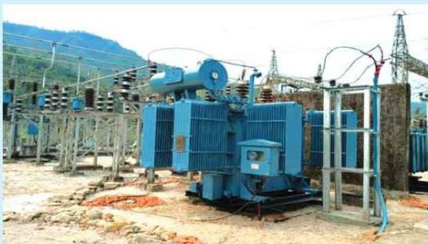
5 MVA 11/66 Transformer at JHP-II
