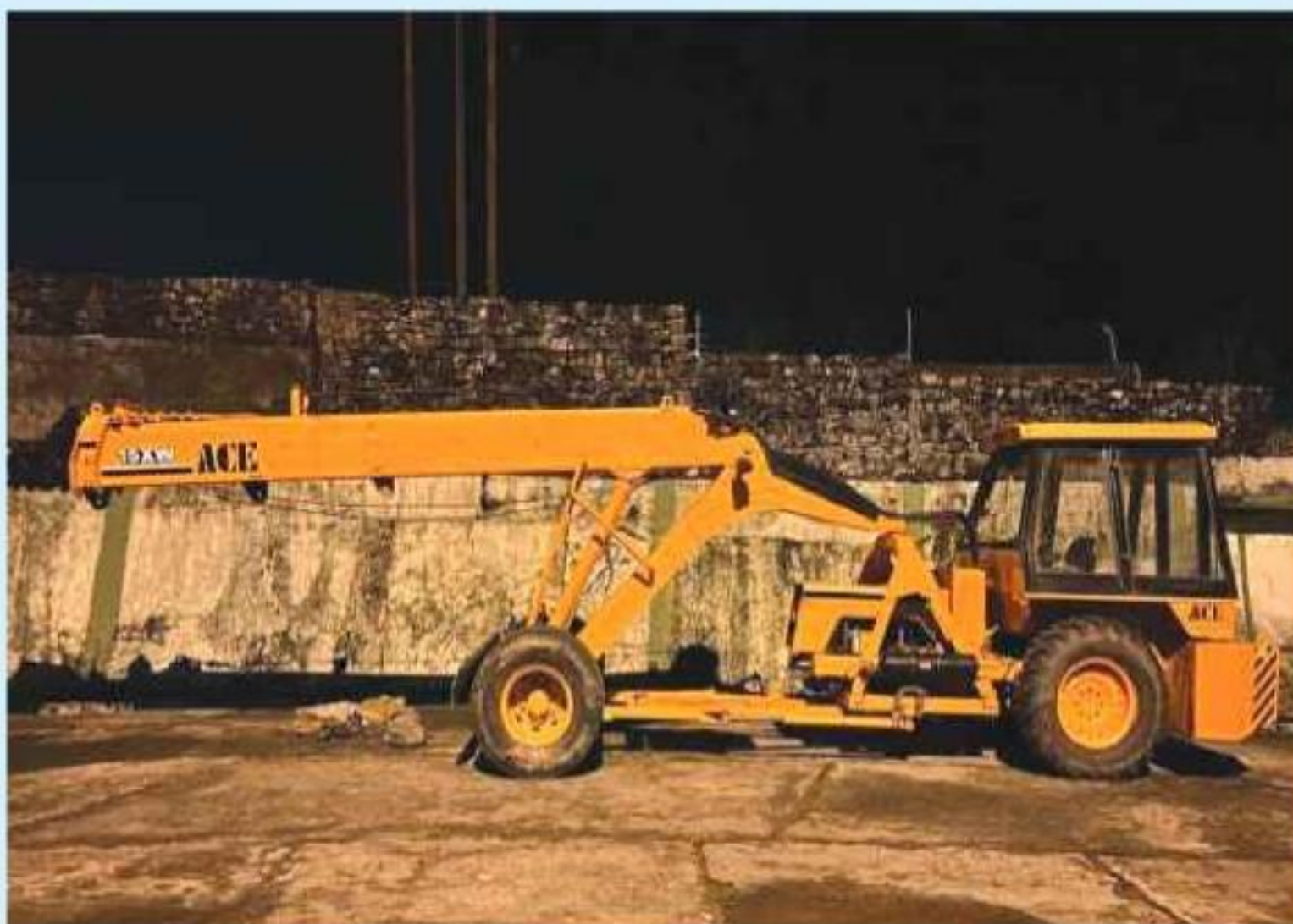
Hydraulic Mobile Crane at Power house, RHP -II
